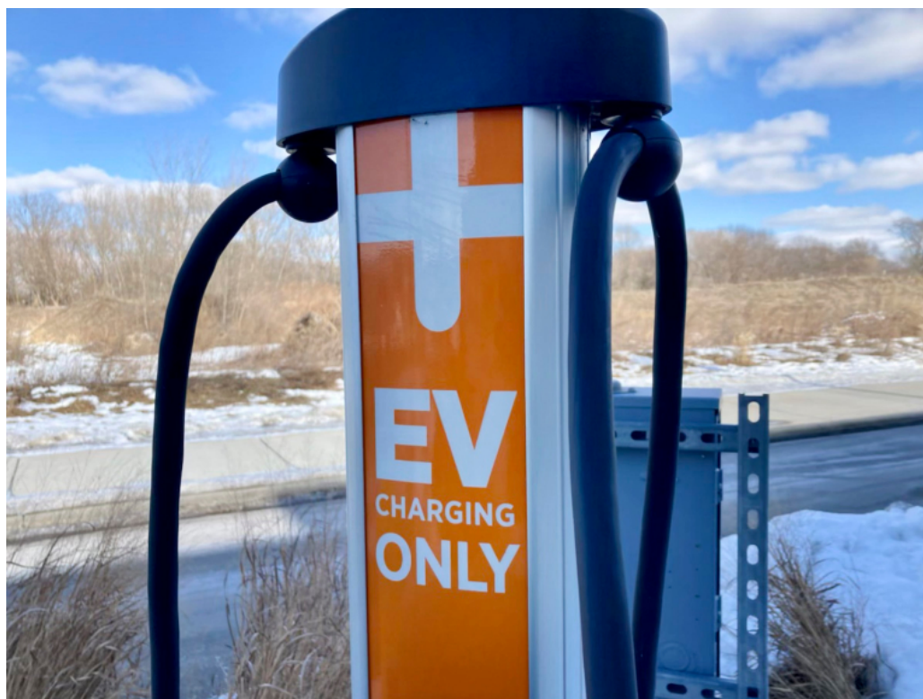
📷 A ChargePoint electric car charging station sits in the parking lot of Garver Feed Mill in Madison, Wis., on Feb. 12, 2022. (Jim Malewitz / Wisconsin Watch)
